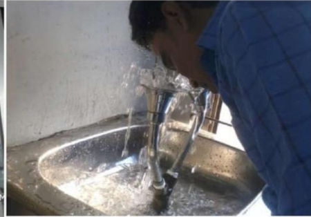
Eye wash Facility at Spot Removing Room
